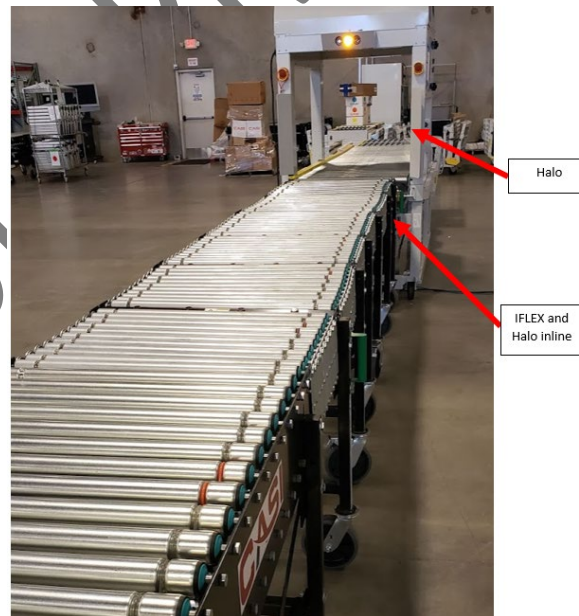
Figure 5 - Move AFLEX Conveyor in Line with Halo Scanner
