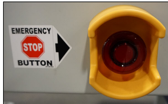
Figure 1 – Emergency Stop (E-Stop) Button
