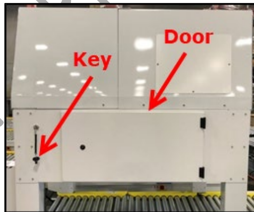
Figure 24 - FAST CASI CORE HMI Cabinet
