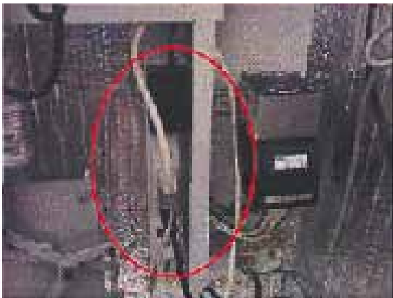
Figure 14. Power strip inside the LPKiosk
