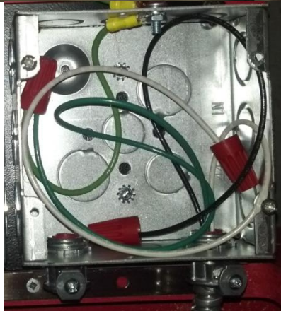
Electrical Wiring Connections
